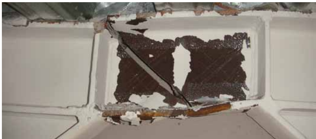
Figure 1: Fractured EBF in Pacific Tower. Courtesy of Sean Gardiner, CPG New Zealand Ltd.
