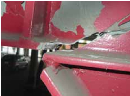
Figure 2: Parking garage with fractured link at lower level EBF. Courtesy of Greg MacRae.
